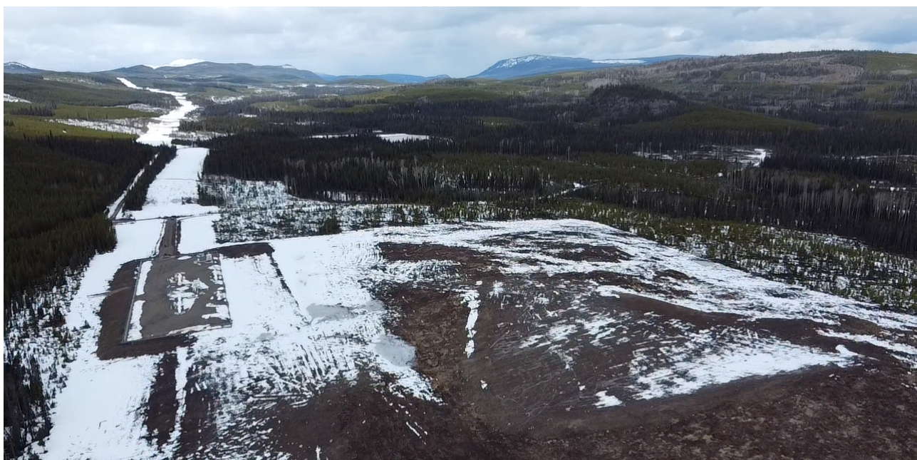
Aerial view of the area cleared to make way for the Parrott Lakes compressor station, April 2025 © Amnesty International (photographer: Alli McCracken)
