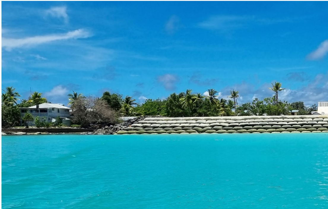
A land reclamation project in Funafuti, predicted to last for approximately 25 years, where sand is dredged from the lagoon and placed in large bags that settle for up to a year before seedlings are planted, then eventually buildings will be constructed and people can move onto the new land. © Amnesty International
