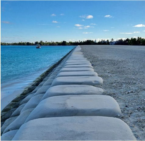
A land reclamation project in Funafuti, predicted to last for approximately 25 years, where sand is dredged from the lagoon and placed in large bags that settle for up to a year before seedlings are planted, then eventually buildings will be constructed and people can move onto the new land. © Amnesty International
