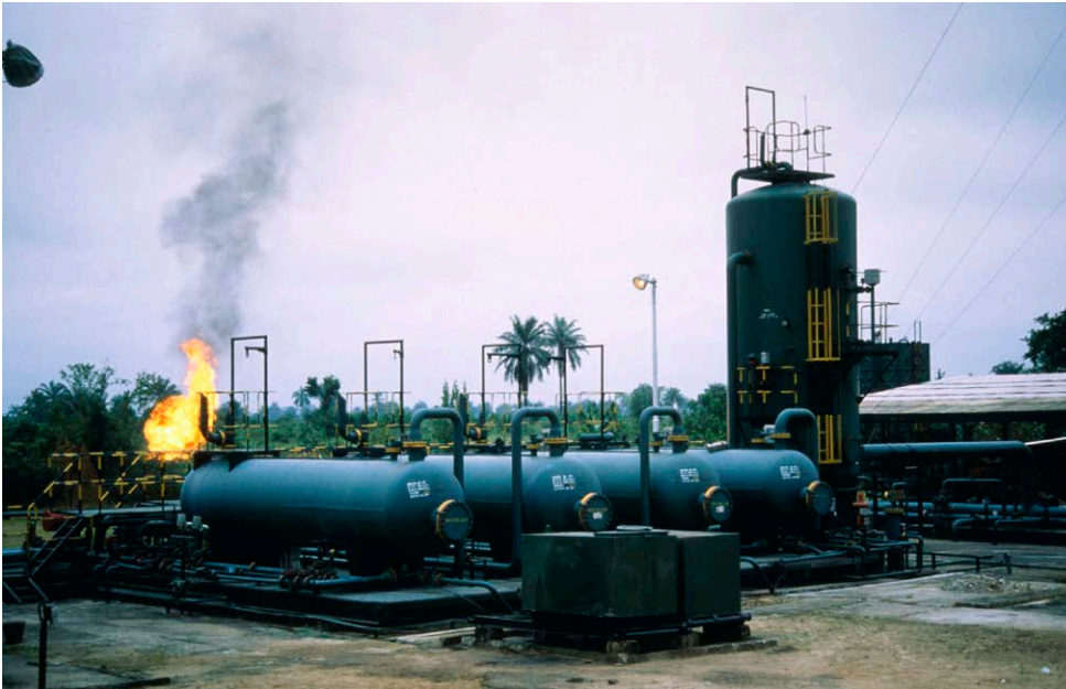
A Shell facility in KoroKoro, Ogoniland, 1994 © Tim Lambon / Greenpeace
